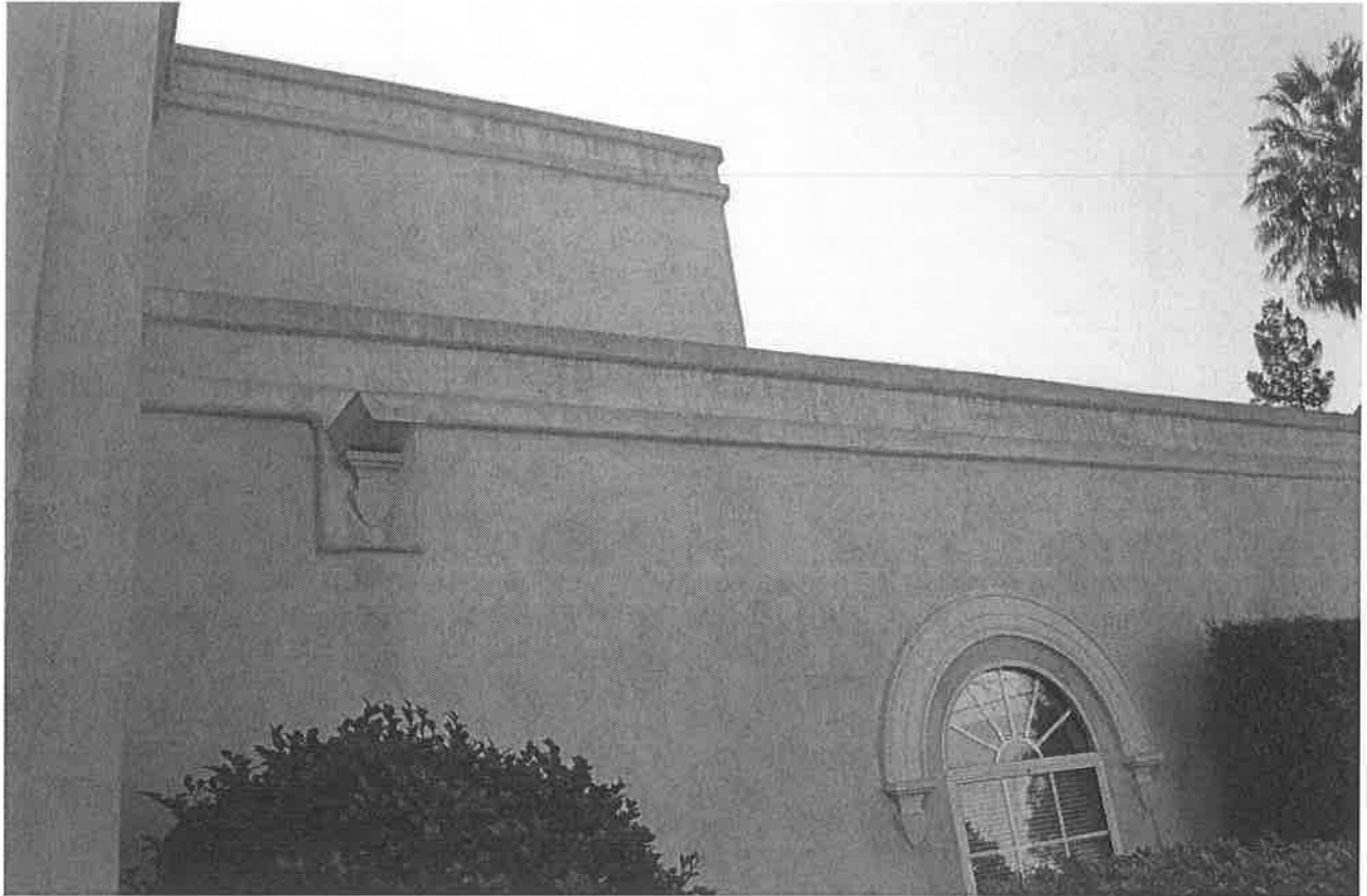
Example of etching of stucco along roof line below horizontal surfaces
